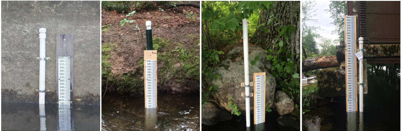
Water level logger locations from left to right: Great Brook, Beaver Brook, lower basin, and Kezar outlet stream. Photo Credit: FBE & KLWA.
